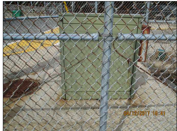
4. Pad-mounted transformer, southwestern portion of Subject Property
