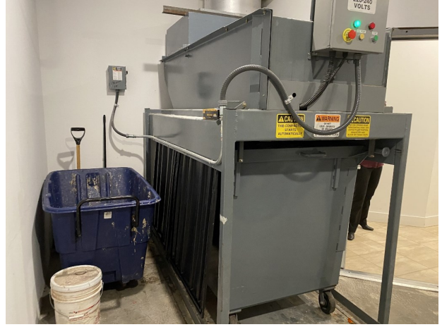
8. View of the trash compactor.
