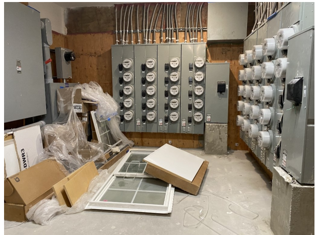
10. View of the electric panels.
