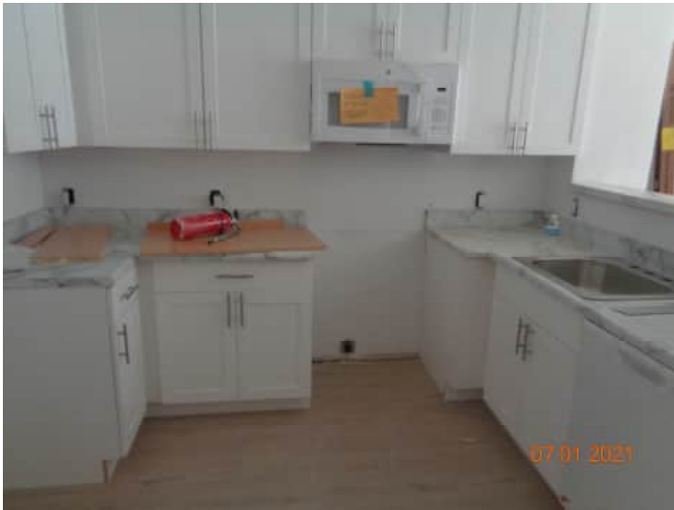
Photo #7 - View of a typical kitchen
