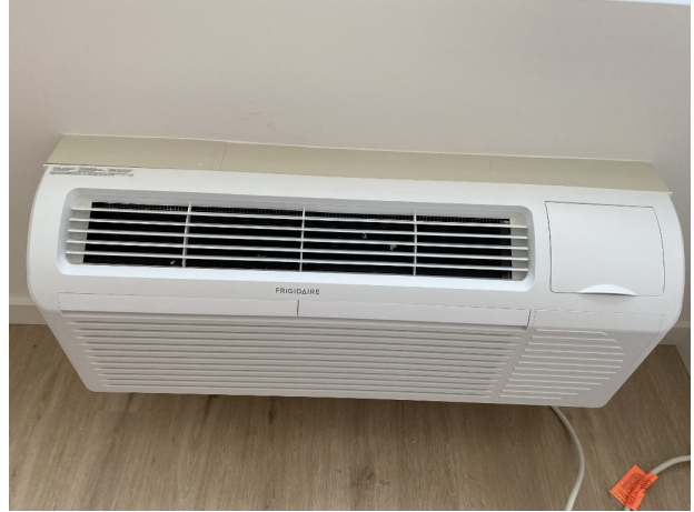
14. View of a typical PTAC unit.
