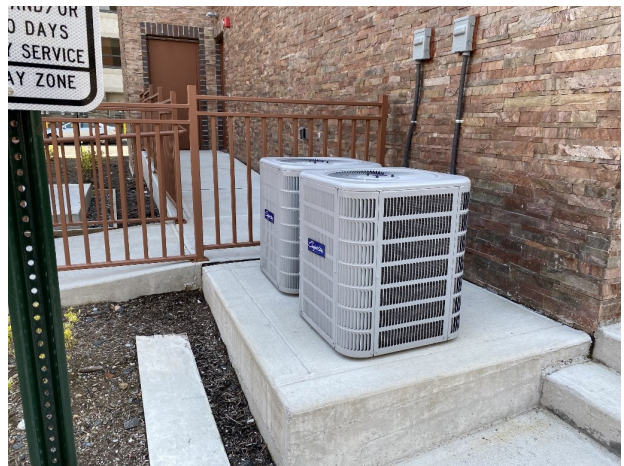
28. View of exterior condenser units.
