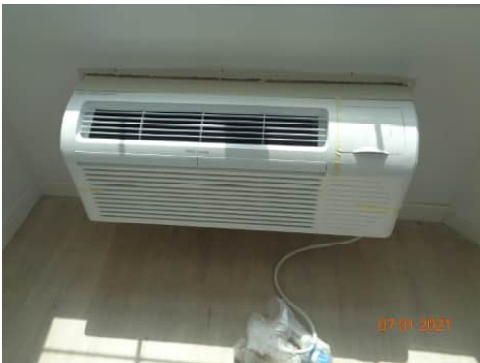
Photo #4 - View of a typical electric PTAC unit
