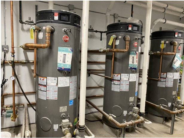
25. View of the natural gas-fired water heaters.
