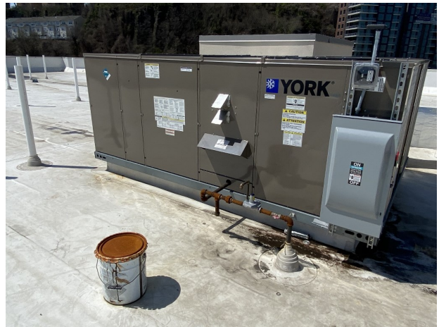
22. View of a rooftop HVAC unit.
