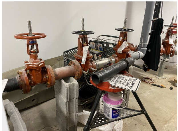
24. View of the fire pump equipment.
