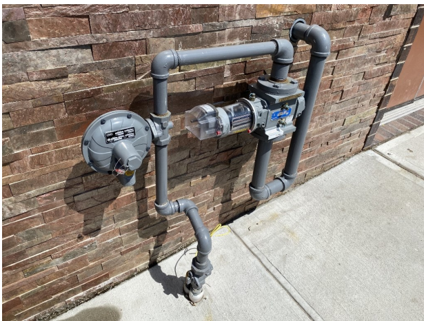
27. View of a natural gas meter.
