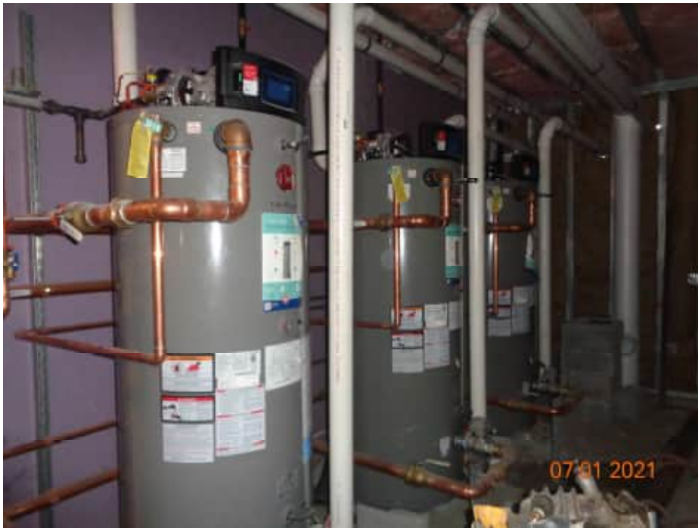
Photo #3 - View of the gas water heaters
