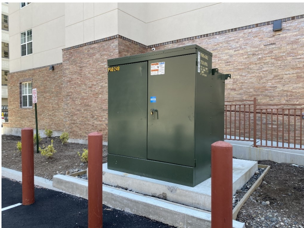
29. View of the pad-mounted transformer.
