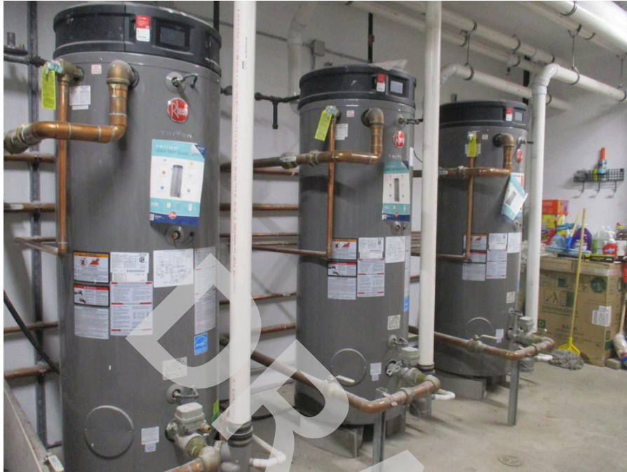
19. Hot water heaters
