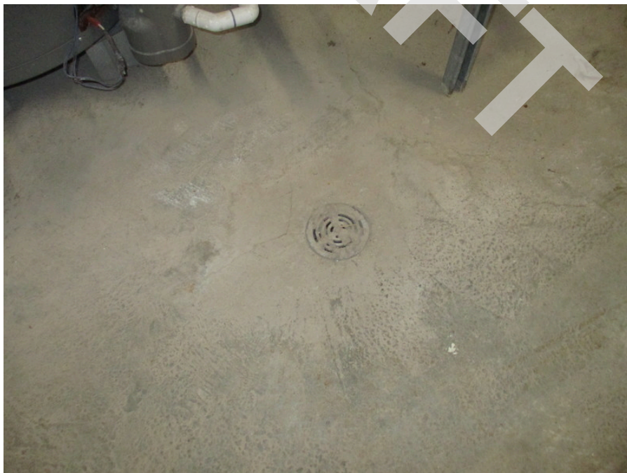
20. Floor drain in boiler room
