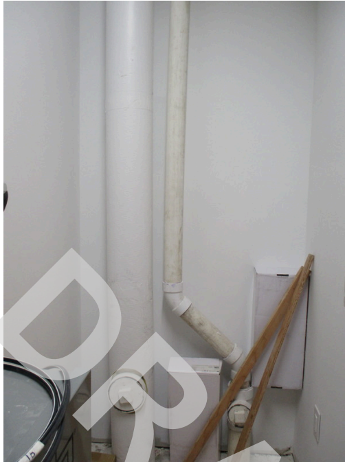
17. Passive sub-slab ventilation pipes
