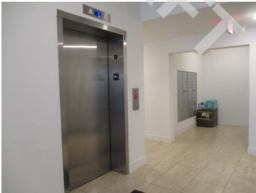
12. Passenger elevator (1 of 2)
