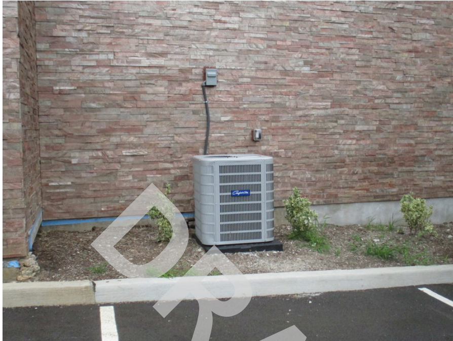
7. Typical condenser unit
