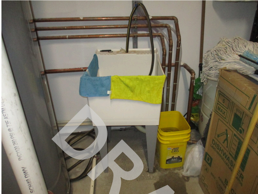
21. Janitorial sink in boiler room
