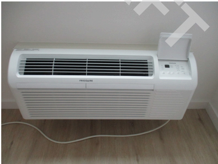
16. Typical AC and Heat Unit (Electrical)
