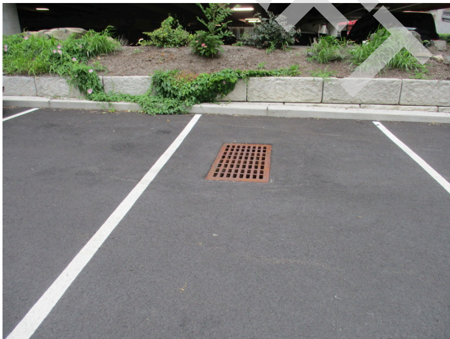
4. Typical stormwater drain
