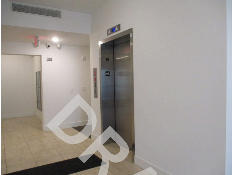
13. Passenger elevator (2 of 2)
