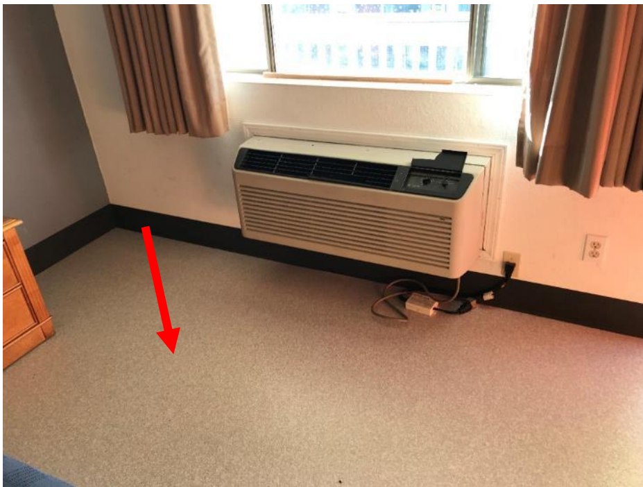
HA No. 1. Grey pebble pattern vinyl floor sheeting, yellow mastic, and grey leveling compound (M)
