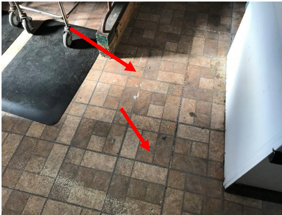
HA No. 16. 12"x 12" red brick pattern vinyl floor tile, clear mastic with debris, black coating, Tan mastic, and brown vinyl floor sheeting(M)
