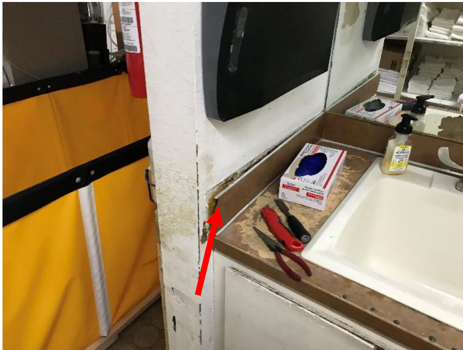
HA No. 18. Brown fiberglass reinforced panel, tan mastic, and joint compound (M)
