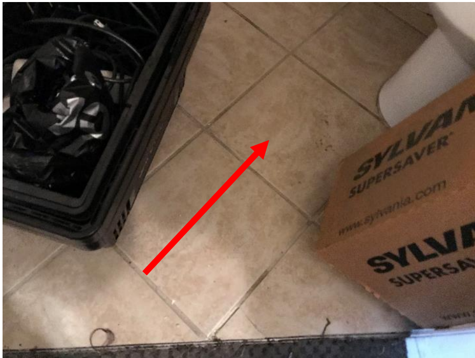
HA No. 36. 12"x 12" tan ceramic floor tile, beige grout, and white mortar (M)
