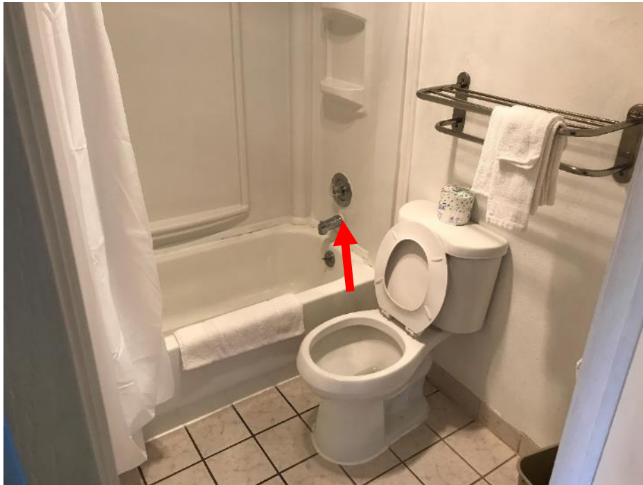
HA No. 10. White sealant, white mastic, and white joint compound (M)
