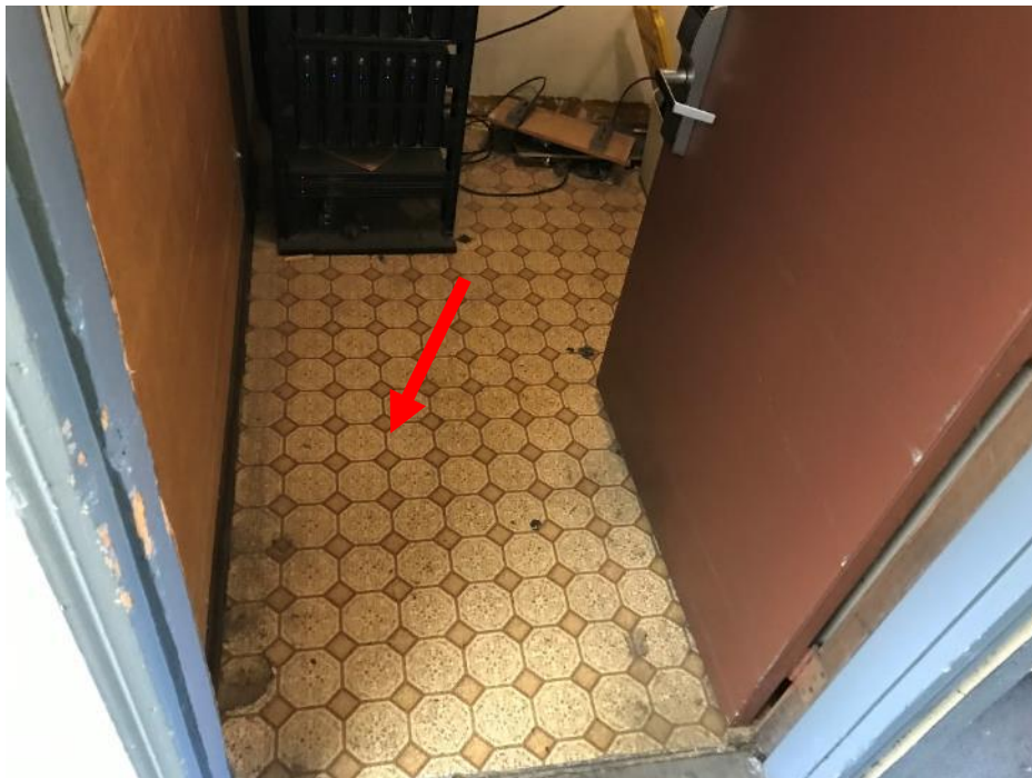
HA No. 11. Tan and brown diamond pattern vinyl floor sheeting with tan mastic (M)
